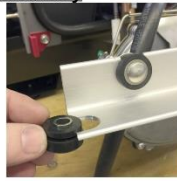
2a-3 Install 2 shock isolators removed from tank onto new fuel module rail.
